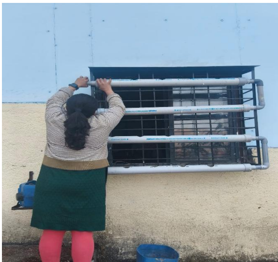
Hydroponics Installation on window
