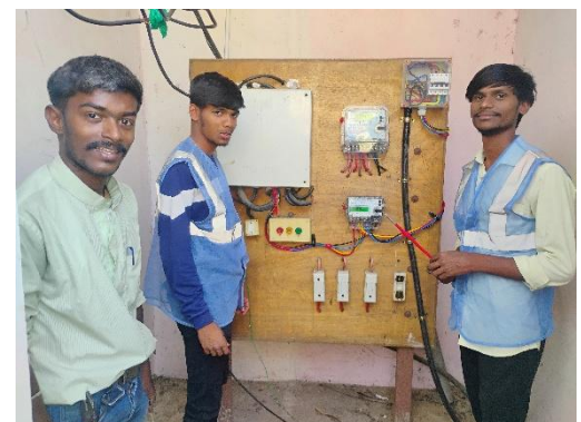
Installed 3 Phase solar system meter
