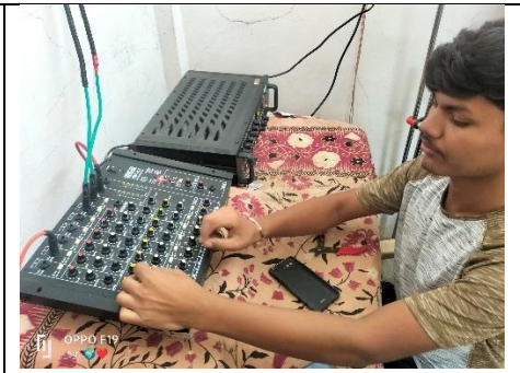
Sound mixer and control system
