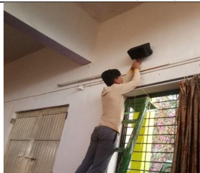
Installing speakers to avoid echo
