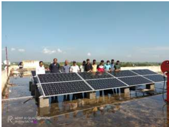
Solar installation @ Mukhai school
