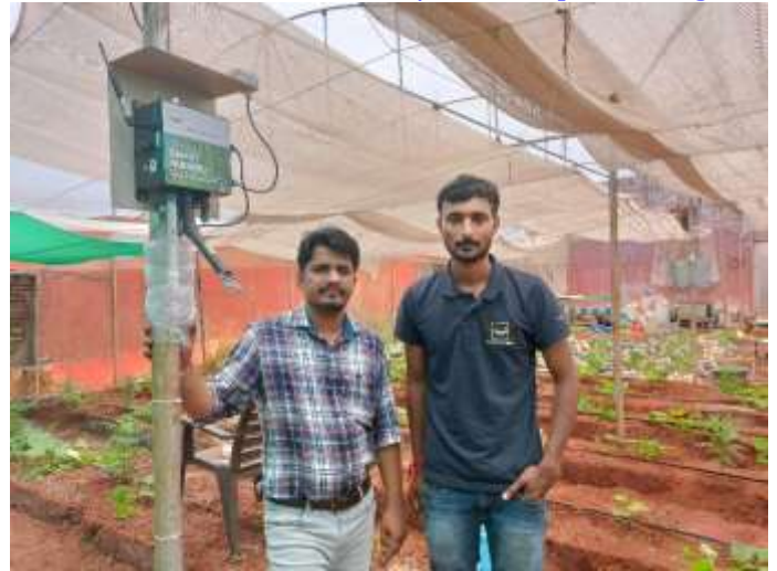
Weather data monitoring Console @polyhouse
