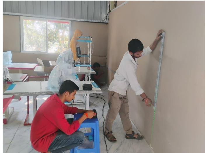
Electrical wiring for Sewing machine room
