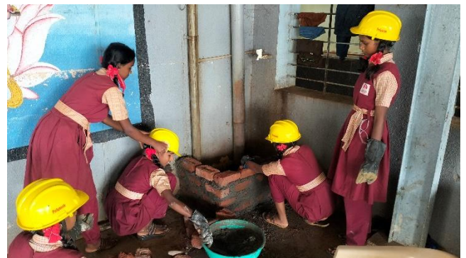
Waghera IBT: Drainage Chamber
