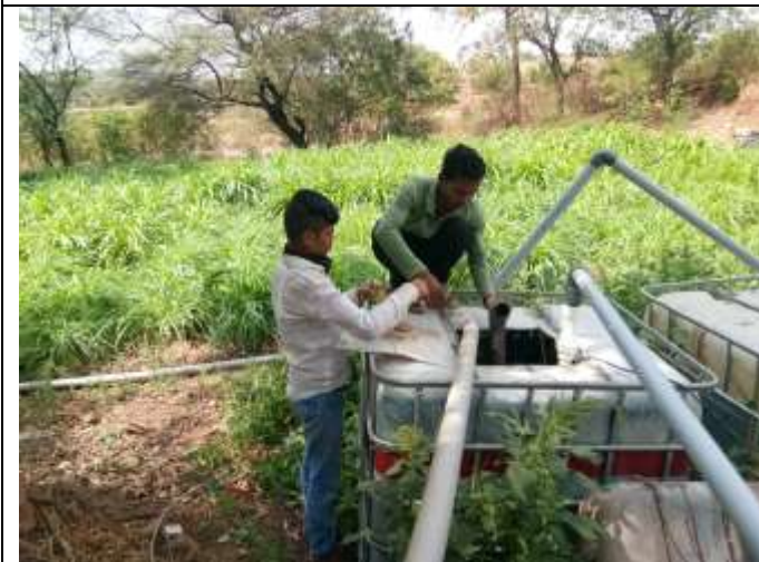
Plumbing @ Grey water recycling system
