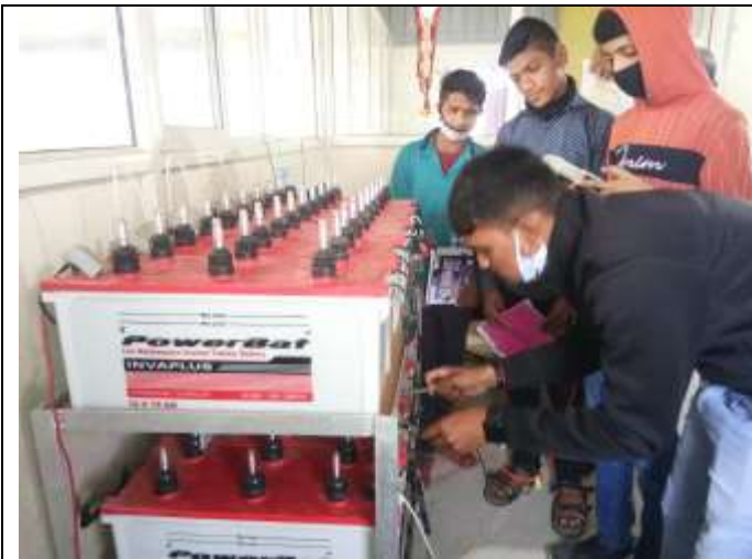
Maintenance of Solar battery
