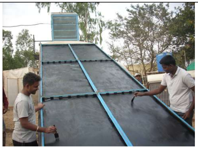
Maintenance of dryer
