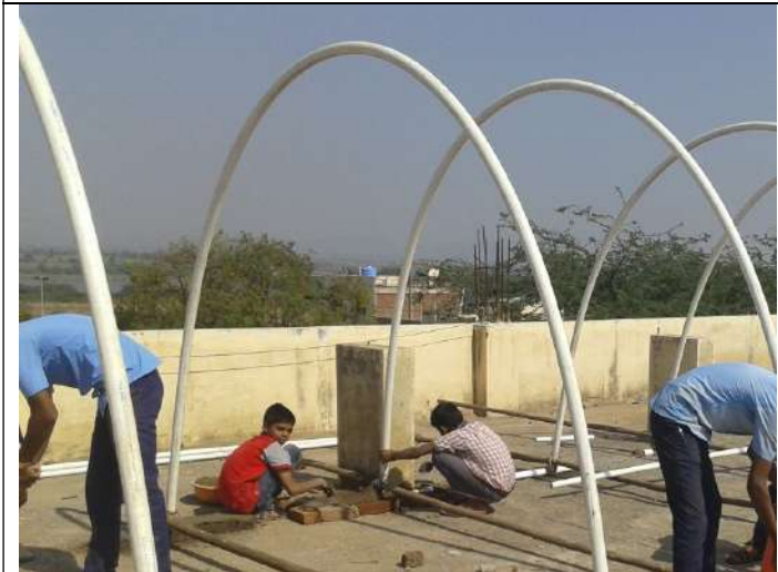
Polyhouse on terrace : IBT @ Shirwal
