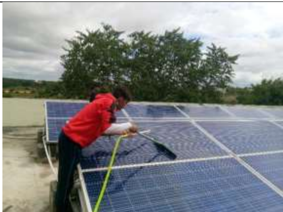
Routine maintenance of solar system
