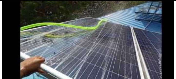
Solar panel cleaning system.
