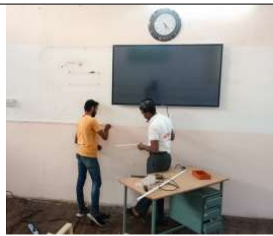
Installing LED TV in the classroom
