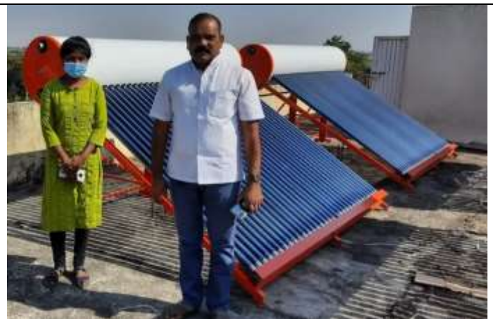
Solar water heater @ Mukhai school
