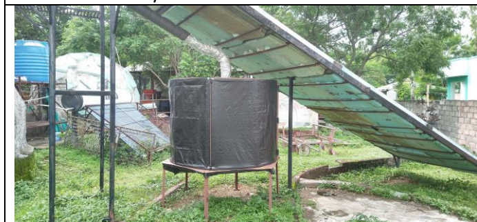
Modified Solar dryer installed
