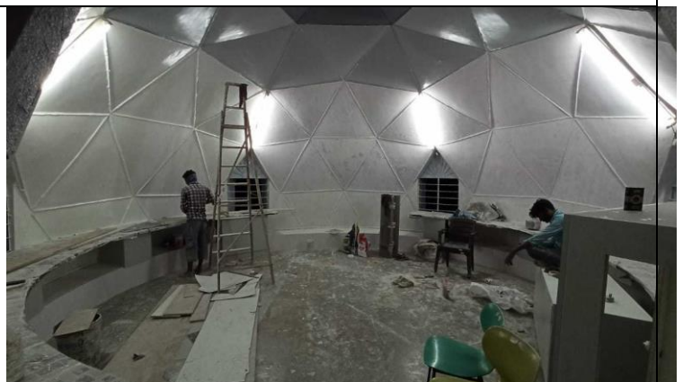
We have started renovation work of DIY Lab with the support of SPA Education Foundation
