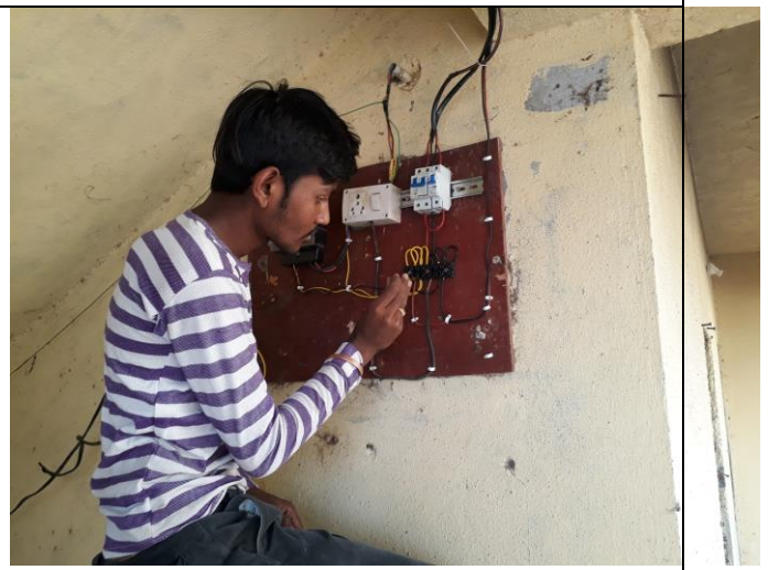
DBRT students : Electrical maintenance
