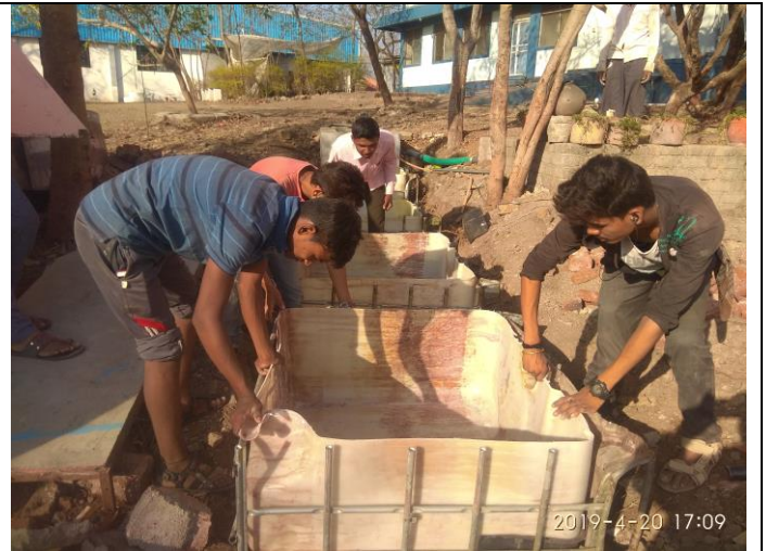
Fabrication Grey water system
