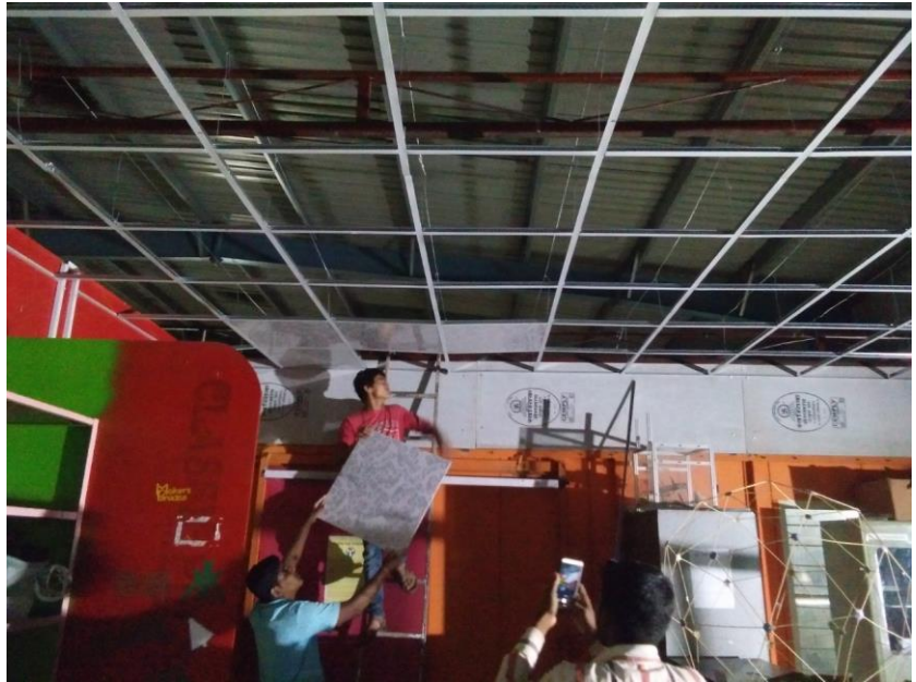
False Ceiling @ Fab Lab
