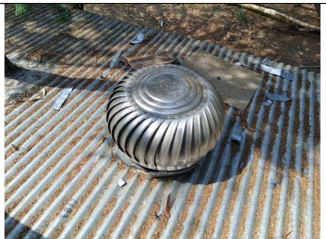
Turbo ventilator on Kitchen Chulha room
