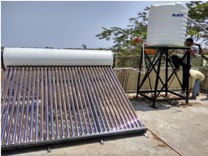
Solar water heater @ boys hostel
