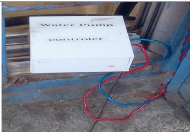
Water pump controller installed in VA campus—made in the Fab Lab
