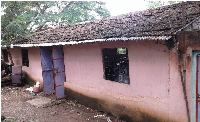
Old Classroom.. lots of memories , It was given 15+ years of service and was housing poultry earlier.
