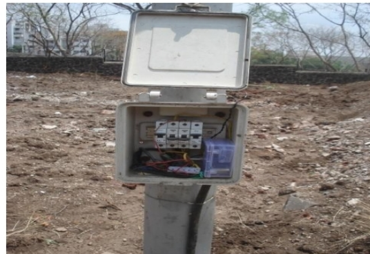
LDR installation at DIY Lab, Pune.
