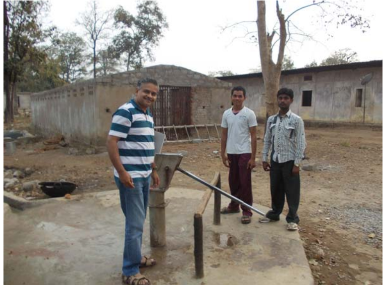
Flooring & handle rest for hand pump : Dugaiguda IBT
