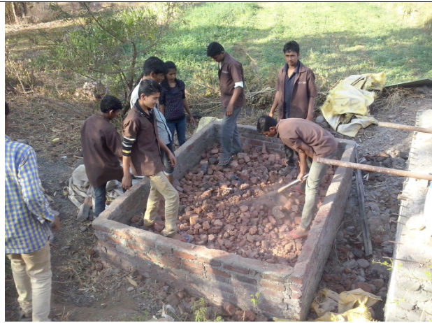
Gray water recycling of staff quarters
