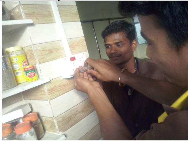
Electrical wiring in new kitchen
